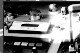
Repeater Unit (Bridge)
